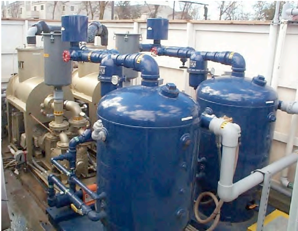
DUAL-PHASE EXTRACTION AND TREATMENT SYSTEM CITRUS HEIGHTS, CA
