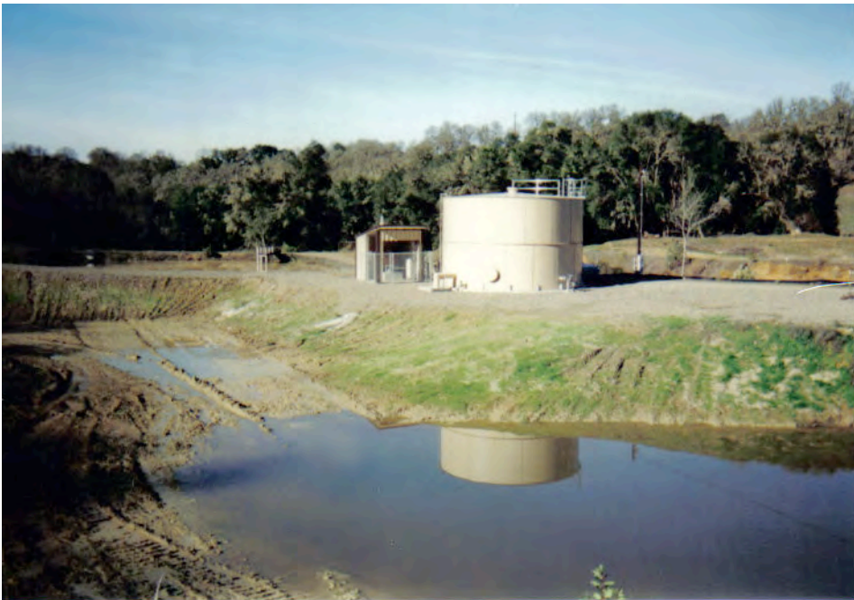
METHANE GAS EXTRACTION AND TREATMENT SYSTEM UKIAH LANDFILL, UKIAH, CA
